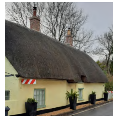
Little Thatch abuts Station Road. The narrow road and heavy traffic use have led to large vehicles damaging the property - hence the need for warning signs.
